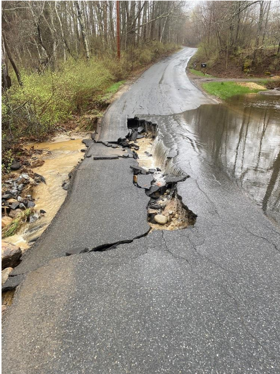
Water overflowing on Daniels Rd
