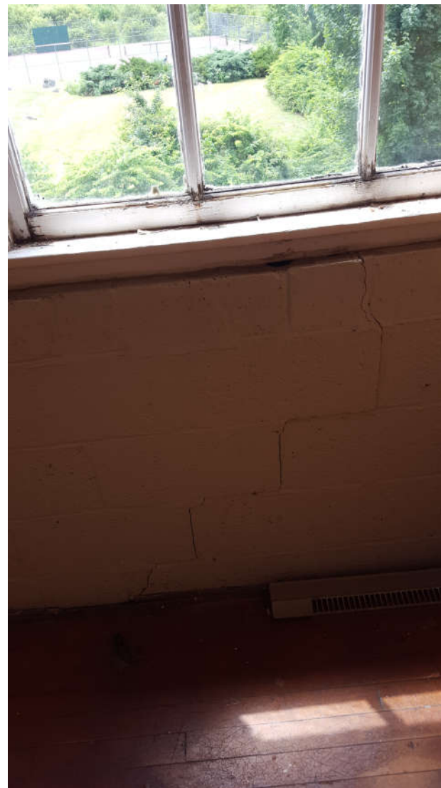
Photo 8 – Cracking at stairwell window 2018
