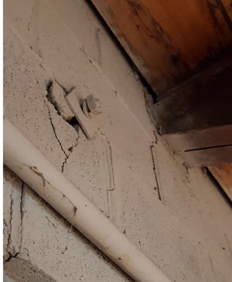
Photo 2 – Crack on North wall 2021
