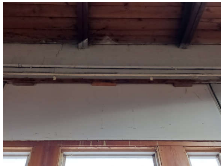
Photo 4 – North wall cracks 2023
