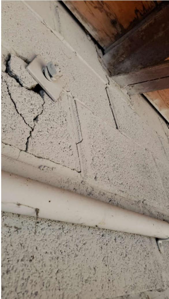
Photo 1 – Crack on North wall 2023
