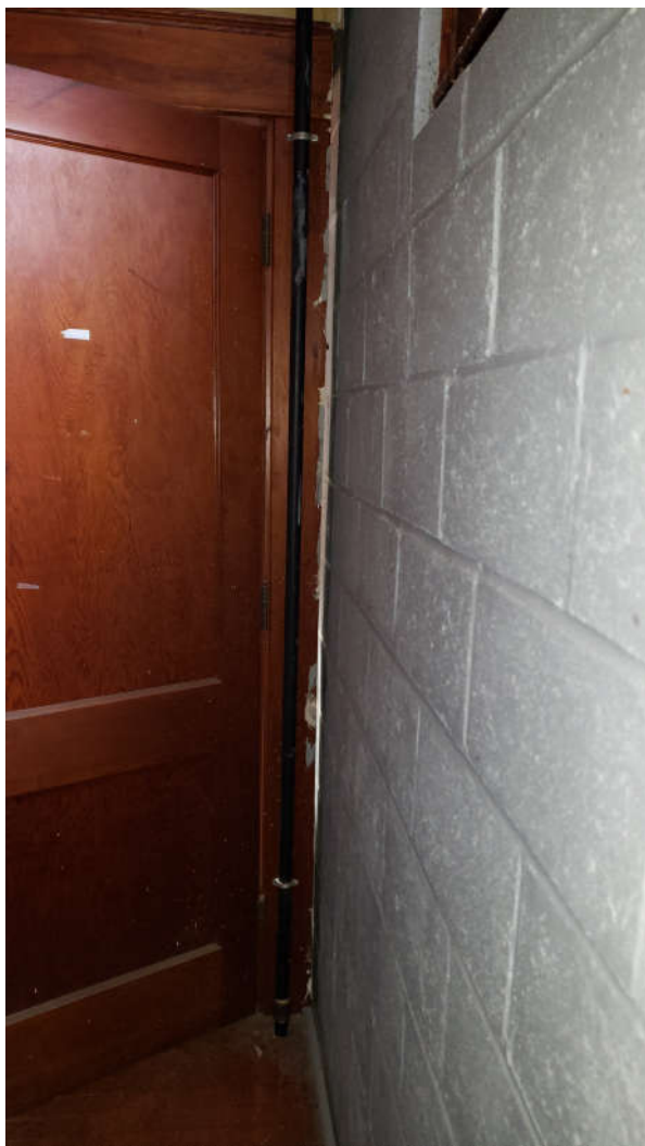
Photo 5 – Displacement at door 2023
