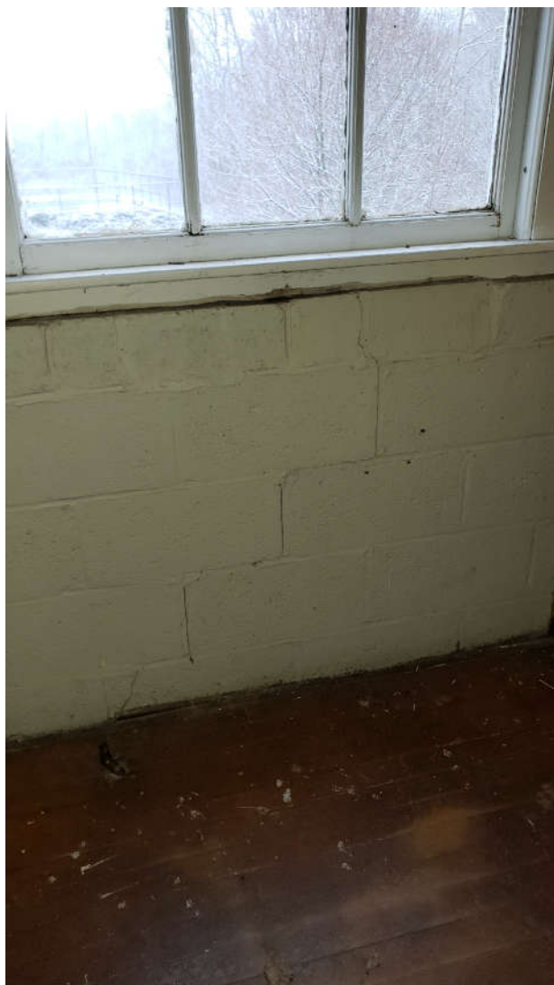
Photo 7 – Cracking at stairwell window 2023
