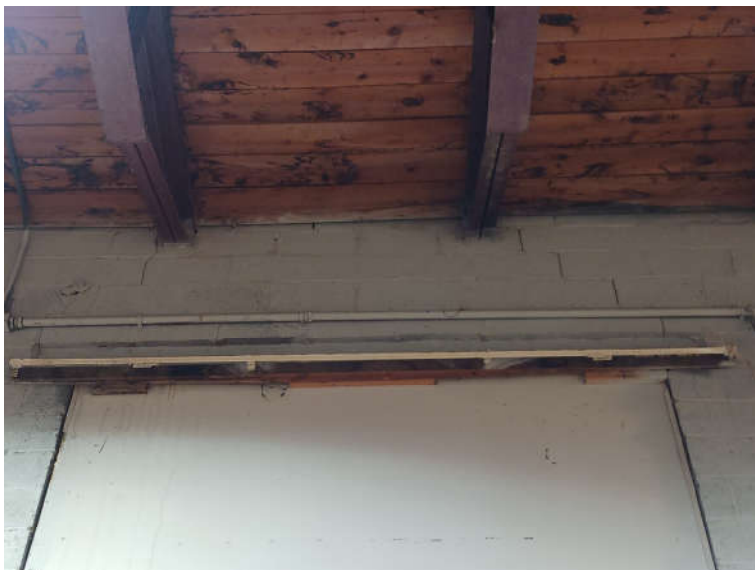
Photo 3 – North wall cracks 2023
